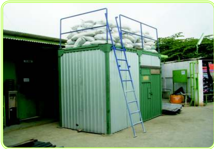
● TEST PUMP ROOM
