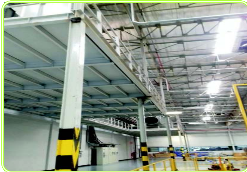
PLATE FORM FOR ELECTRICAL PANEL
