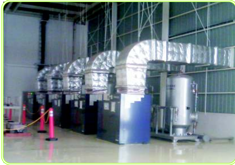
HEAT TRANSFER DUCTING
